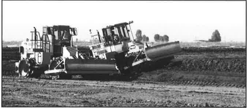
KDW's 815F compactor and another rented unit at work on a Bay Area jobsite
